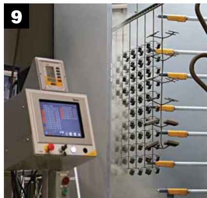
9 Powder is applied with 18 automated and 2 manual spray guns. Compressed process air is dried to -35°F Dew Point for superior adhesion.
